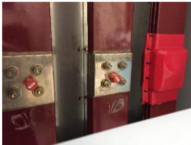
Figure 17: Example Temperature Sensor under Insulation Boots
