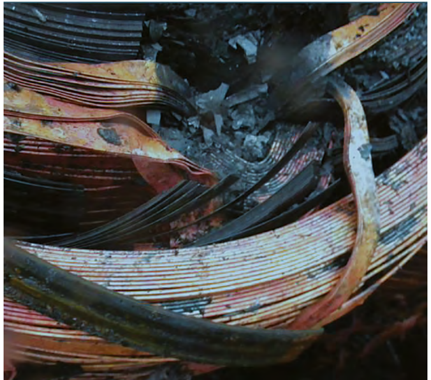
Figure 2. B-phase winding showing radial buckling damage with no shorted turns
