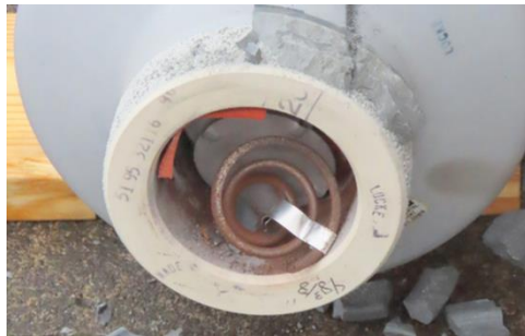
Rusted components from moisture
