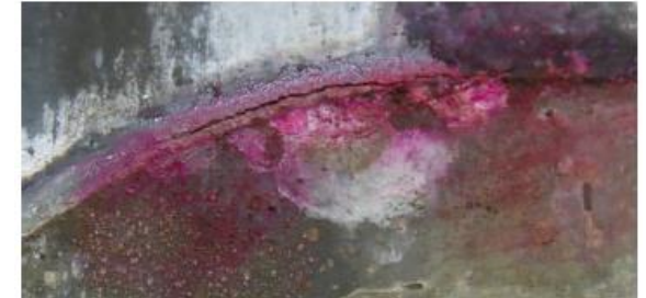
Dye test confirmed an opening at the top diaphragm
