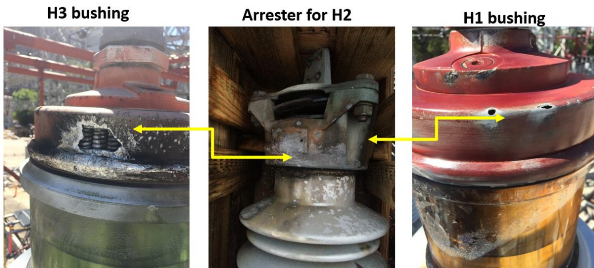
H2 Arrester Venting Event Caused H1 and H3 Bushing Failures Figure 1
