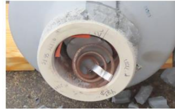
Rusted components from moisture.
