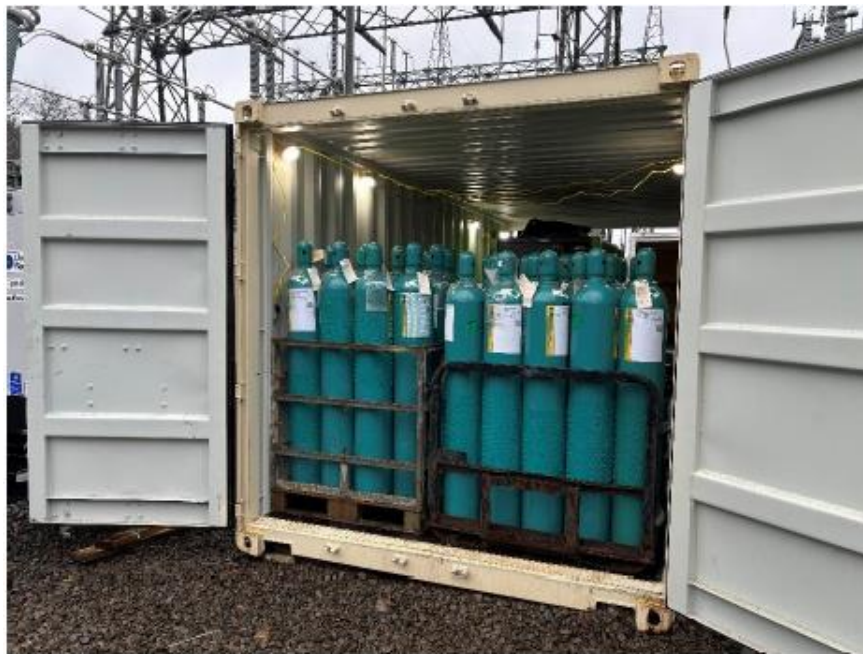
Gas Bottles in Heated Conex Container Figure 9
