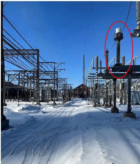
a) 13.8kV Power Line
