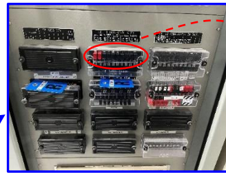
b) Relay panel in control room
